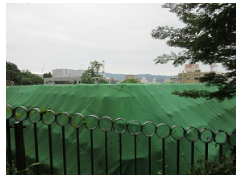
Piles of flexible containers covered with green sheets which have a chimney to let out the air.
